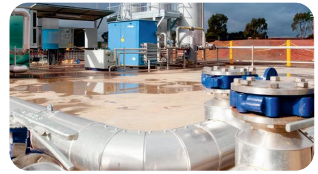
Our Melton Recycled Water Plant
