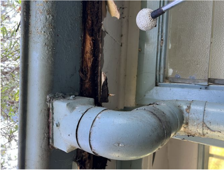
Image comments: Timber rot carpentry
