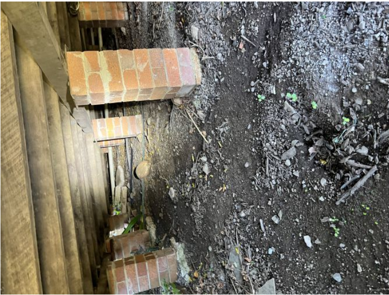
Image comments: Leaning piers
