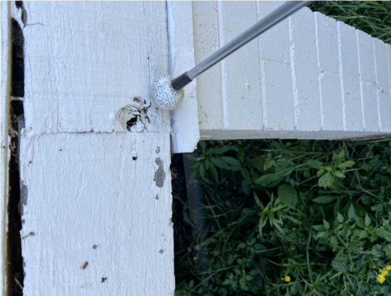
Image comments: Timber rot carpentry
