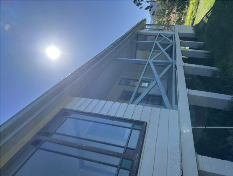
Image comments: Saggign guttering
