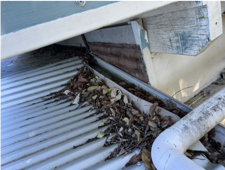
Image comments: Sagging rusted guttering into box section
