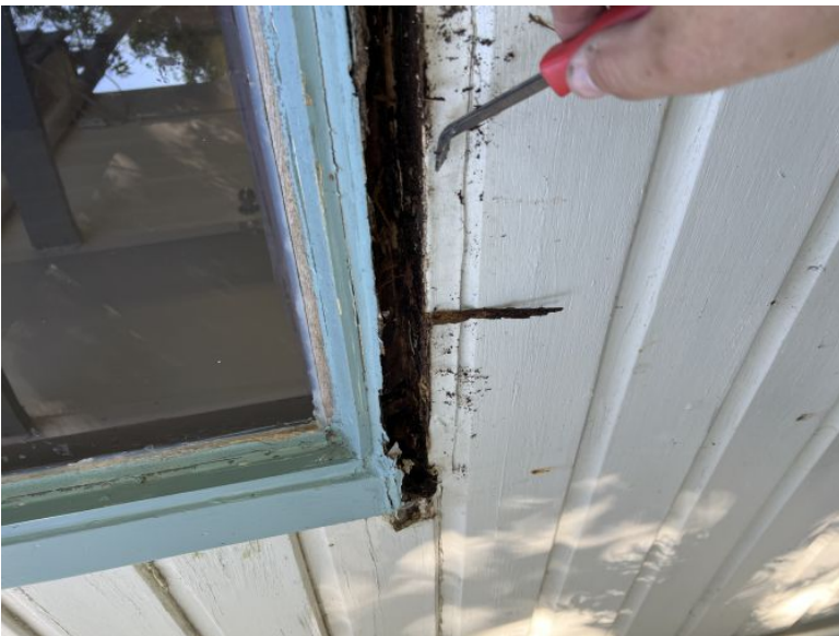
Image comments: Timber rot carpentry
