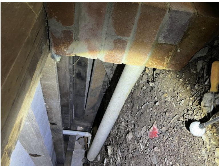
Image comments: Limited crossflow ventilation
