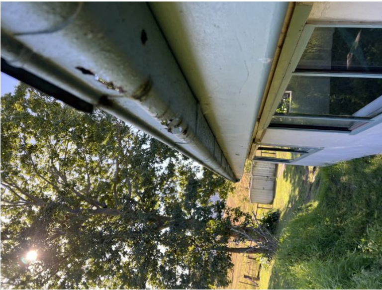
Image comments: Rusted out guttering
