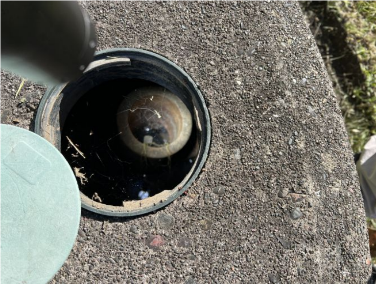
Image comments: Septic tank
