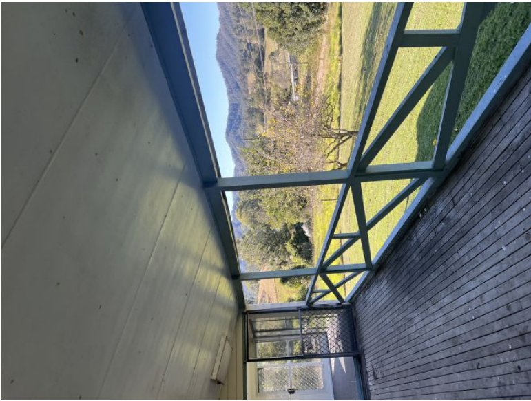
Image comments: Water marks ceiling
