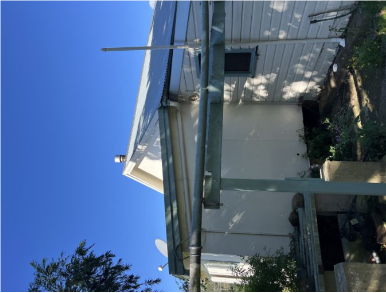
Image comments: Inadequate DPs and guttering
