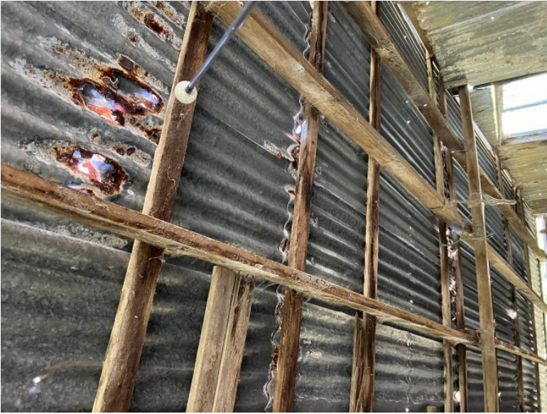
Image comments: Dairy building span of timbers sags
