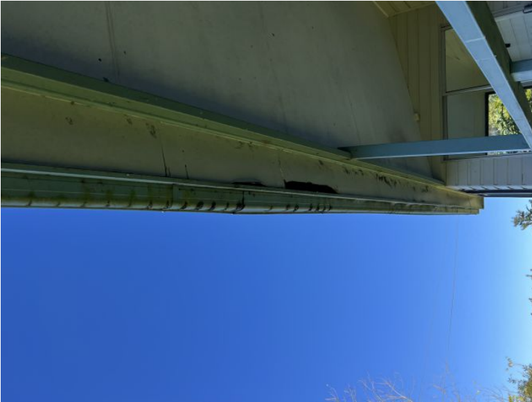
Image comments: Timber rot eaves
