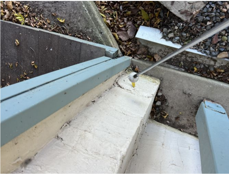
Image comments: Timbers to ground
