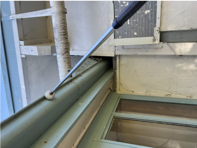
Image comments: Sagging rusted guttering into box section
