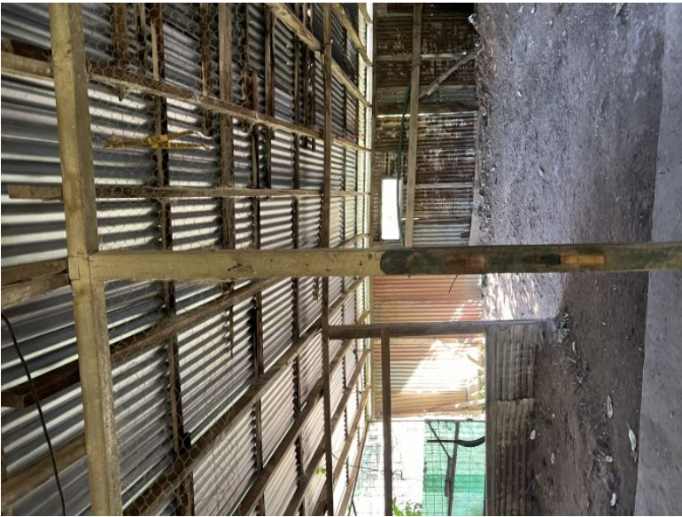
Image comments: Dairy building span of timbers sags
