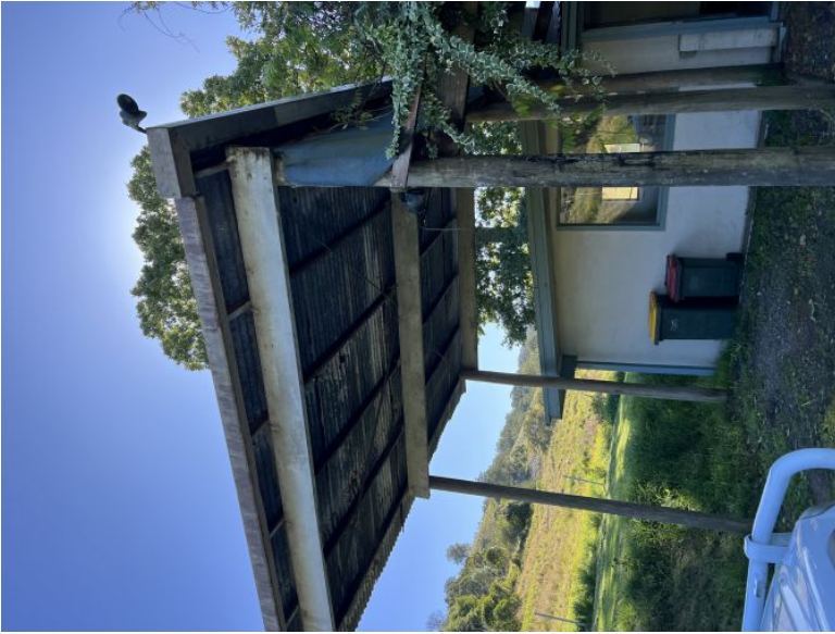
Image comments: Carport rusted out guttering
