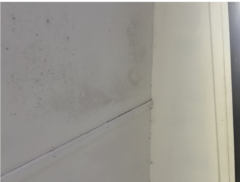
Image comments: Water marks ceiling
