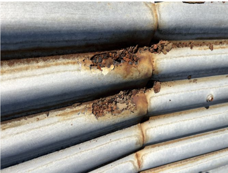
Image comments: Rusted roofing iron
