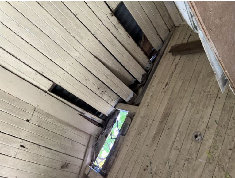
Image comments: Widespread damage
