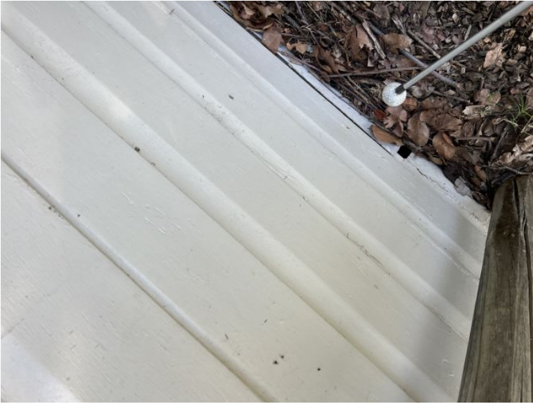
Image comments: Timbers to ground
