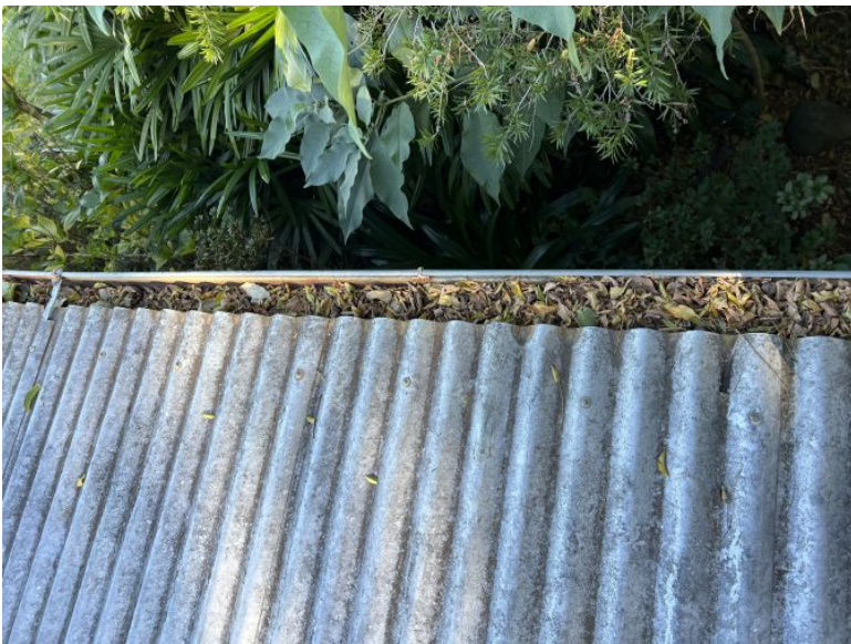
Image comments: Rusted guttering full of debris
