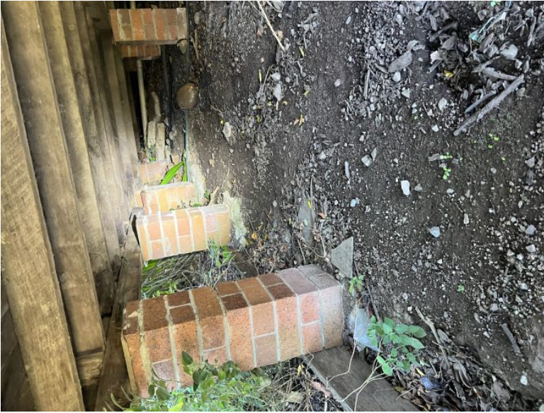
Image comments: Leaning piers
