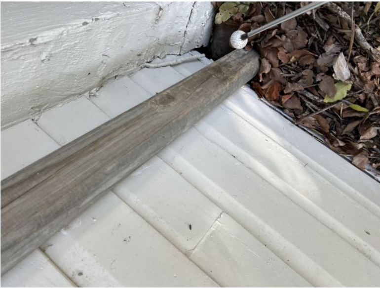
Image comments: Timbers to ground
