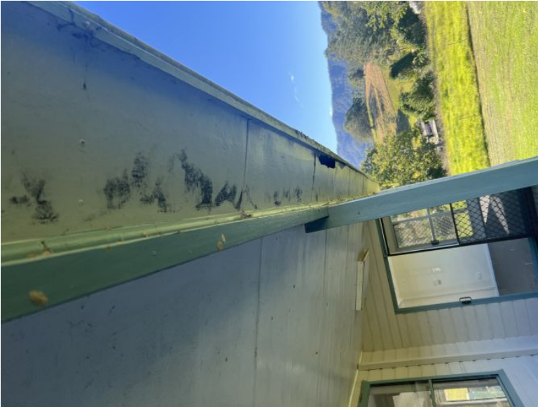
Image comments: Water marks ceiling
