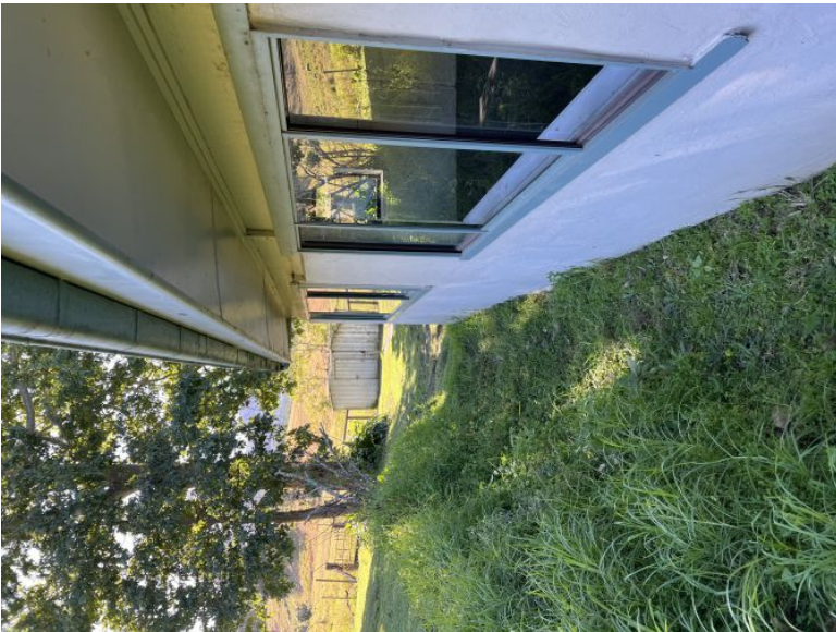
Image comments: Runoff to rear of dwelling to subfloor
