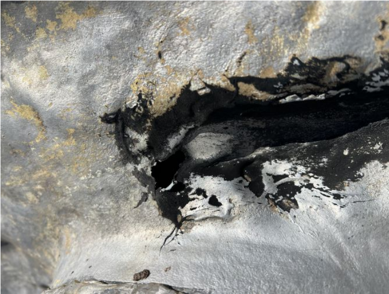
Image comments: Hole in flashing
