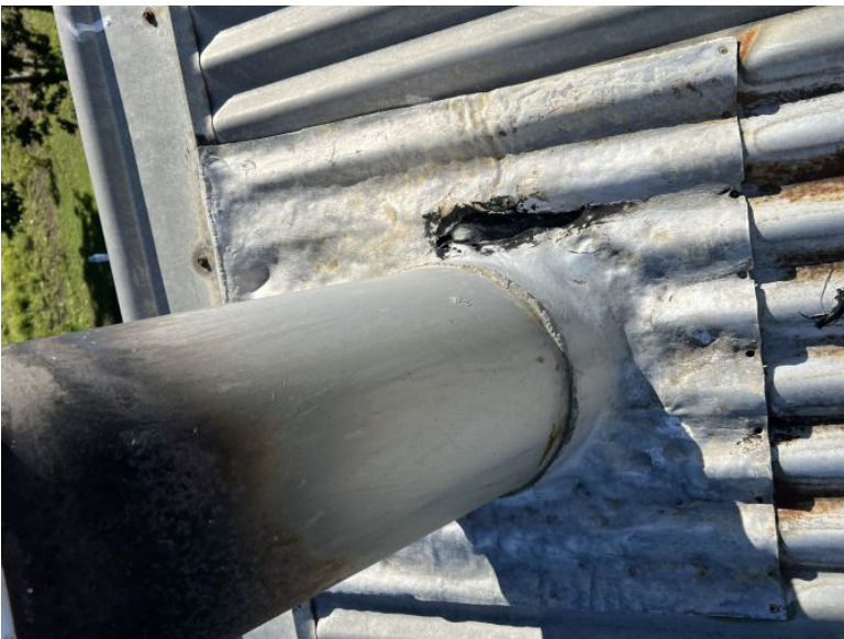
Image comments: Hole in flashing
