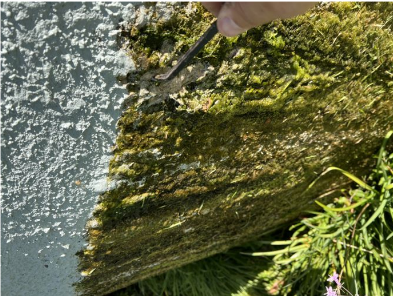
Image comments: Leaking water tank around crack
