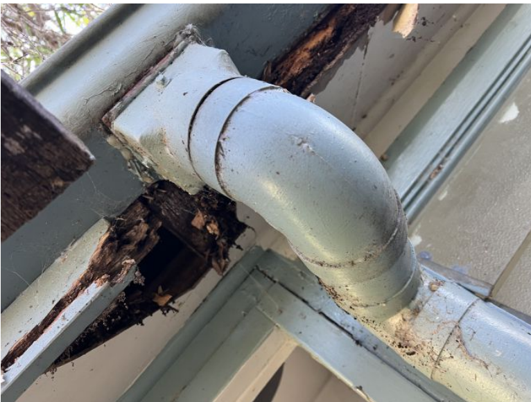
Image comments: Timber rot eaves
