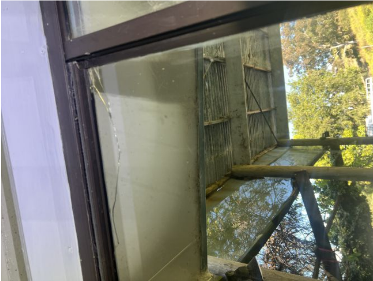
Image comments: Cracked glass
