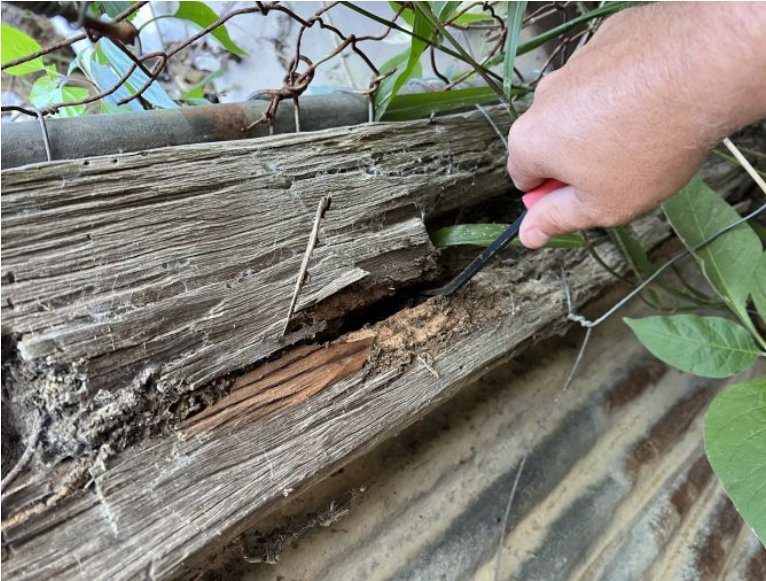
Image comments: Widespread damage
