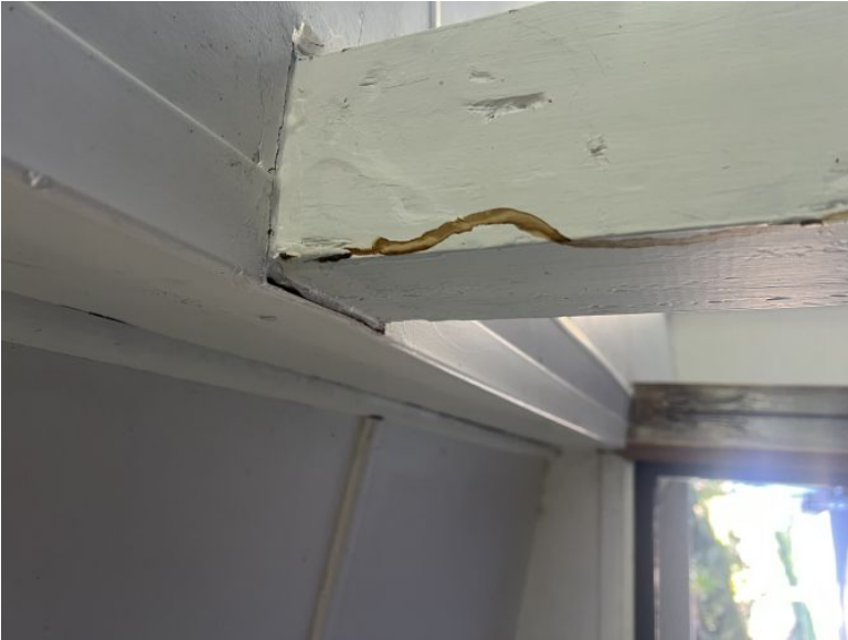
Image comments: Water marks ceiling
