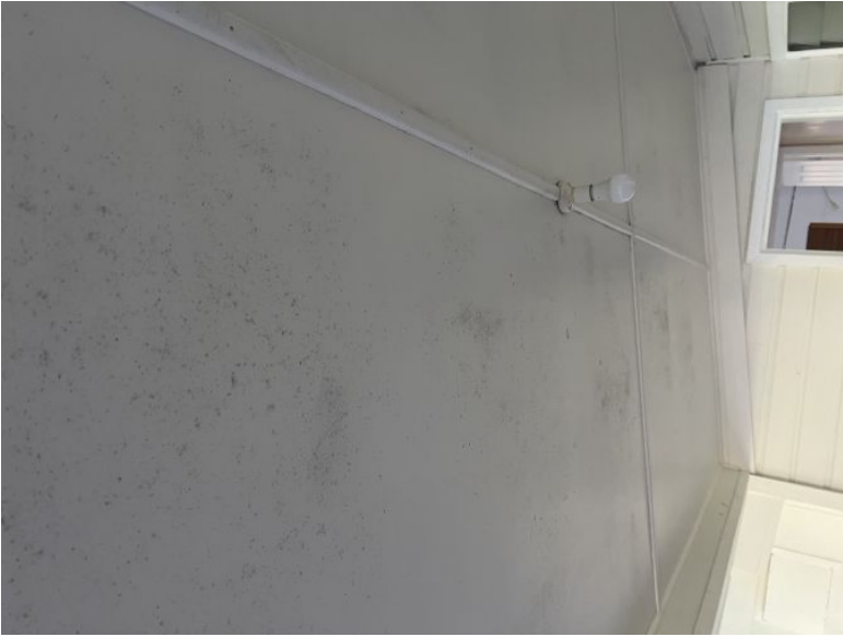
Image comments: Water marks ceiling
