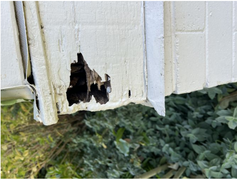
Image comments: Timber rot carpentry
