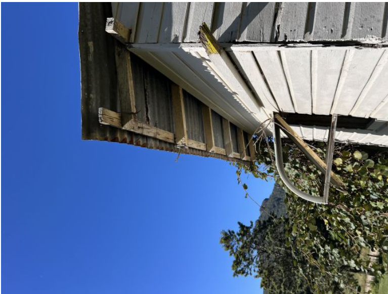
Image comments: Dairy no guttering
