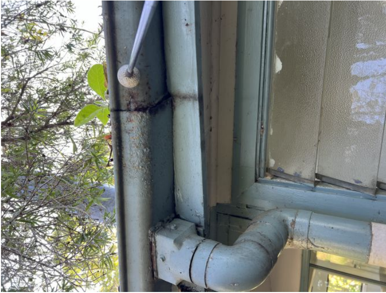
Image comments: Rusted out guttering
