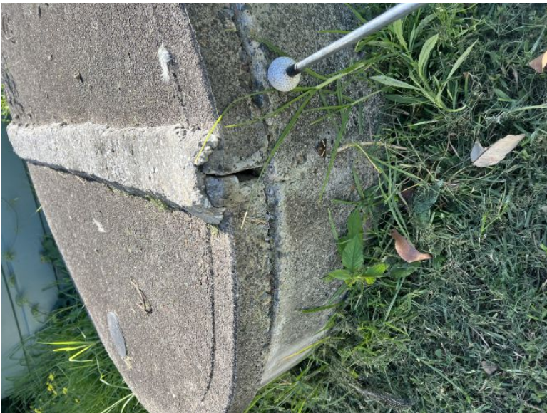
Image comments: Unsealed septic tank
