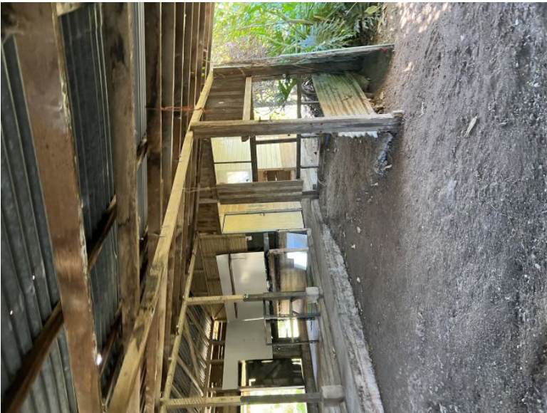
Image comments: Dairy building span of timbers sags
