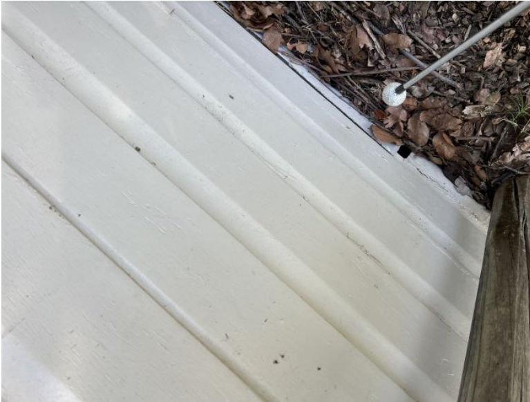
Image comments: Timber rot carpentry
