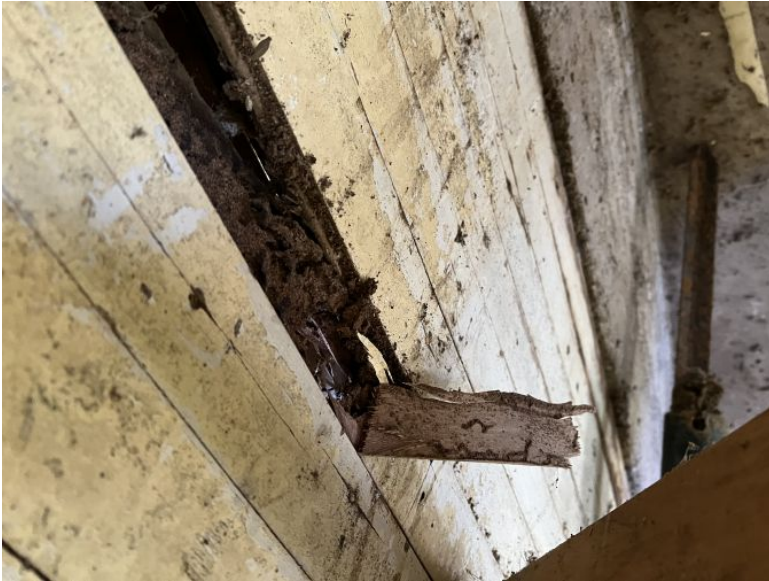
Image comments: Widespread damage
