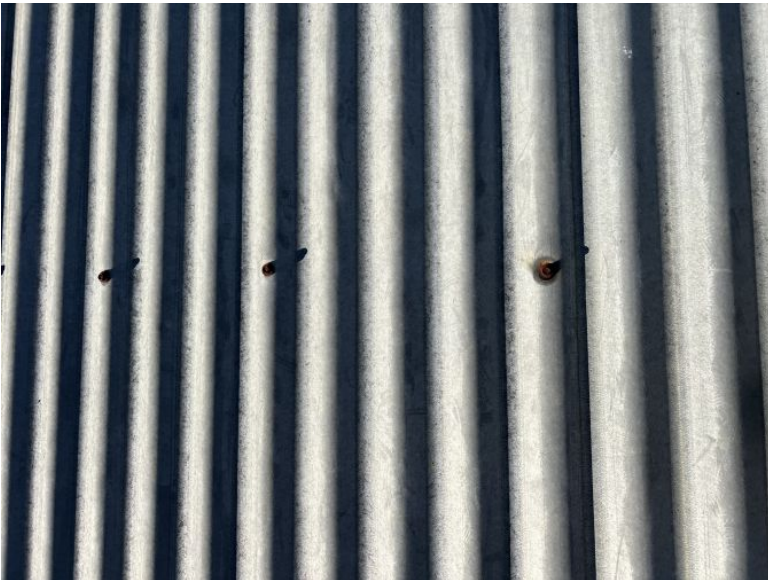
Image comments: Rusted roofing screws
