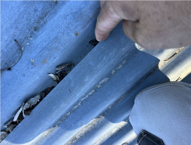
Image comments: Loose roofing iron
