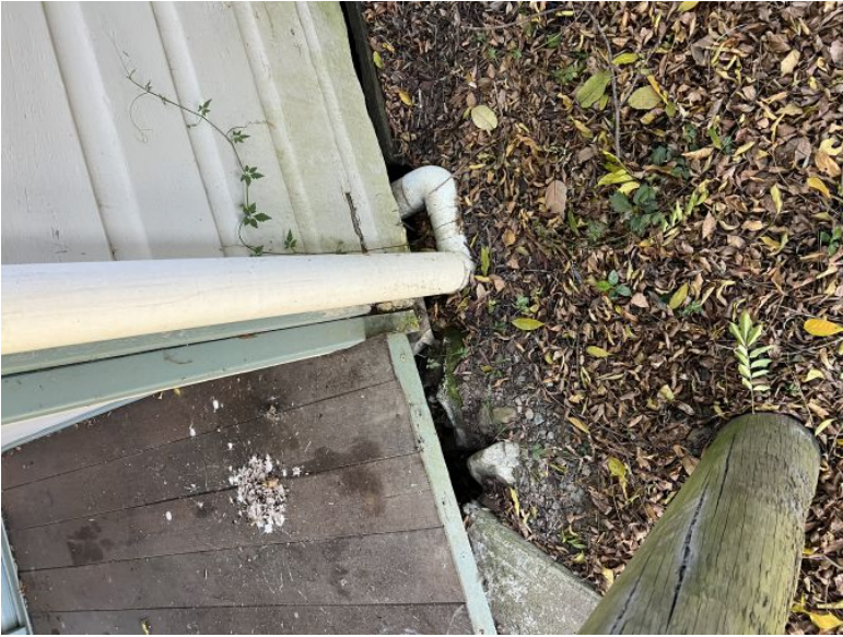
Image comments: Timbers to ground
