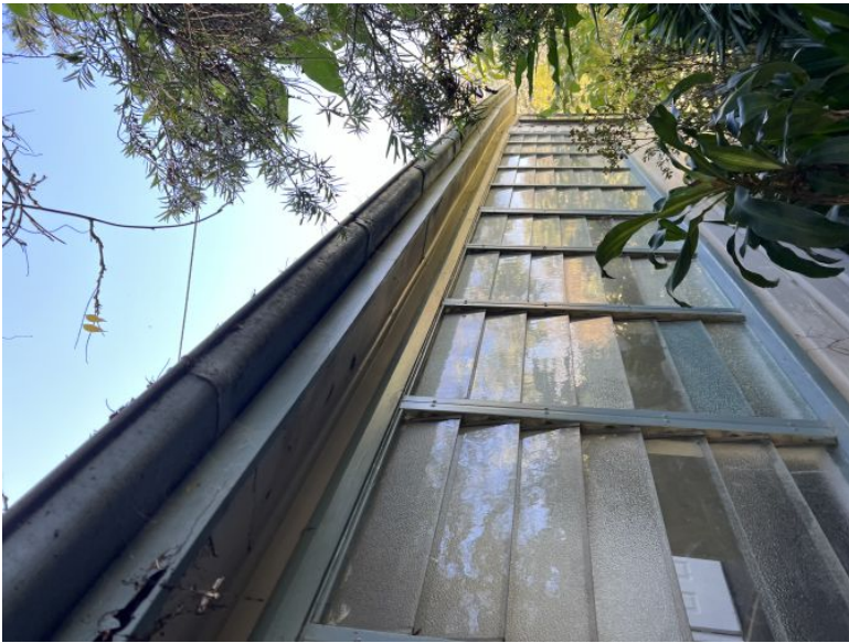
Image comments: Rusted out guttering
